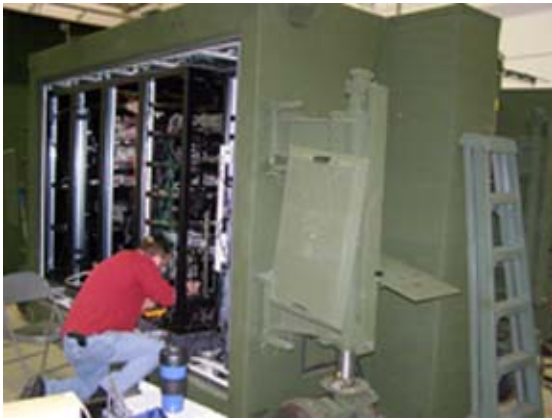
Internal View of Central Equipment Hut
