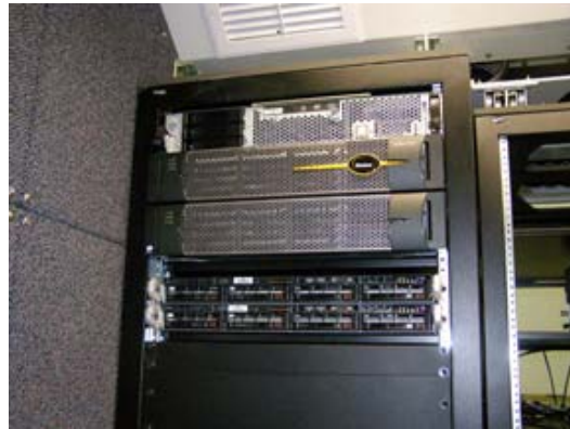
DICES VoIP Equipment
